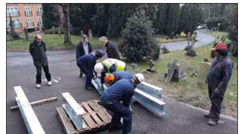
The crew, expertly marshalled by Oggy, lifting one of the steel beams into the tower
